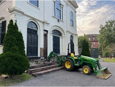
The arm of the bulldozer helping to remove the front stairs of the Meetinghouse so they can be repaired
