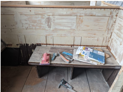
Inside one of the 106 box pews, that is being repaired, sanded, and repainted
