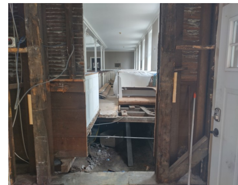
Hole cut in the front wall of the Meetinghouse that will be part of the new handicapped accessible entranceway.
