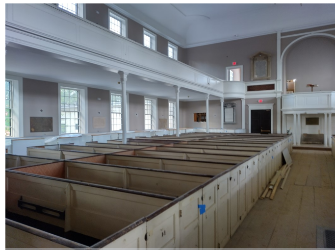
The interior of the Meetinghouse after the removal of the scaffolding. As you can see, the walls and ceiling have been repaired and painted.
